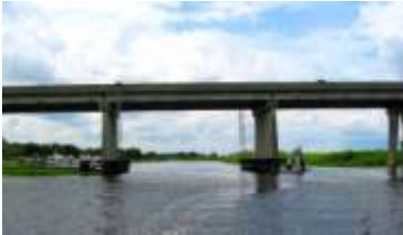
Hwy 415 bridge over St. Johns River near entrance to Lake Monroe, Sanford
